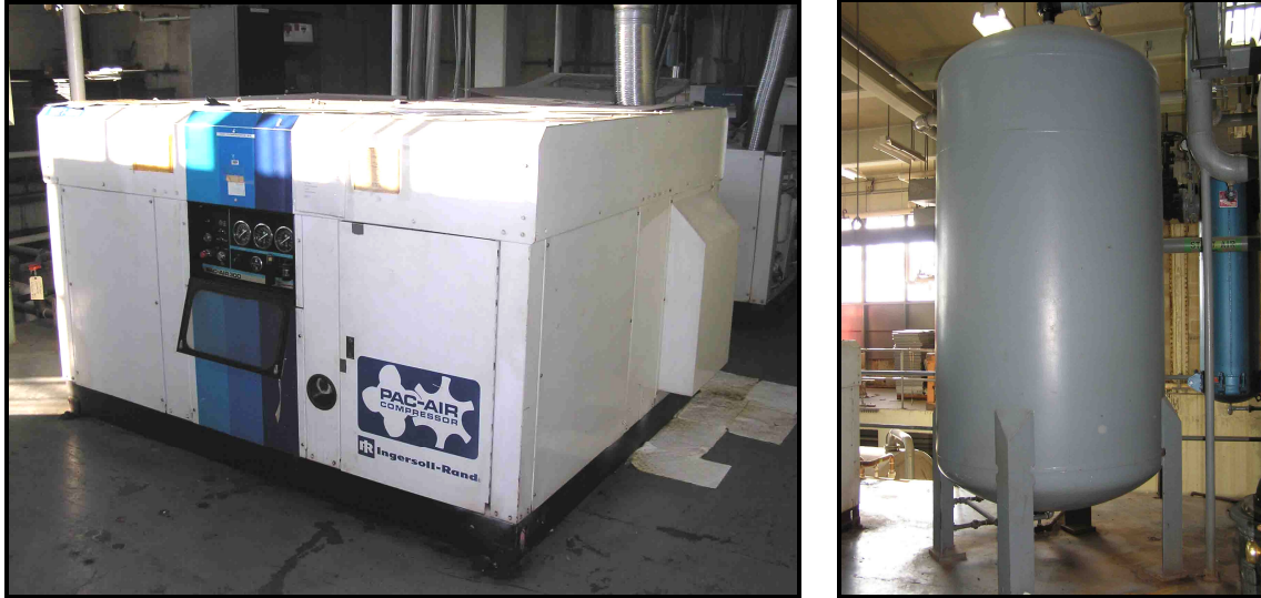
Figure 20. Photographs of the air compressors (left) as well as the receiver tank (right), located in the compressor room
