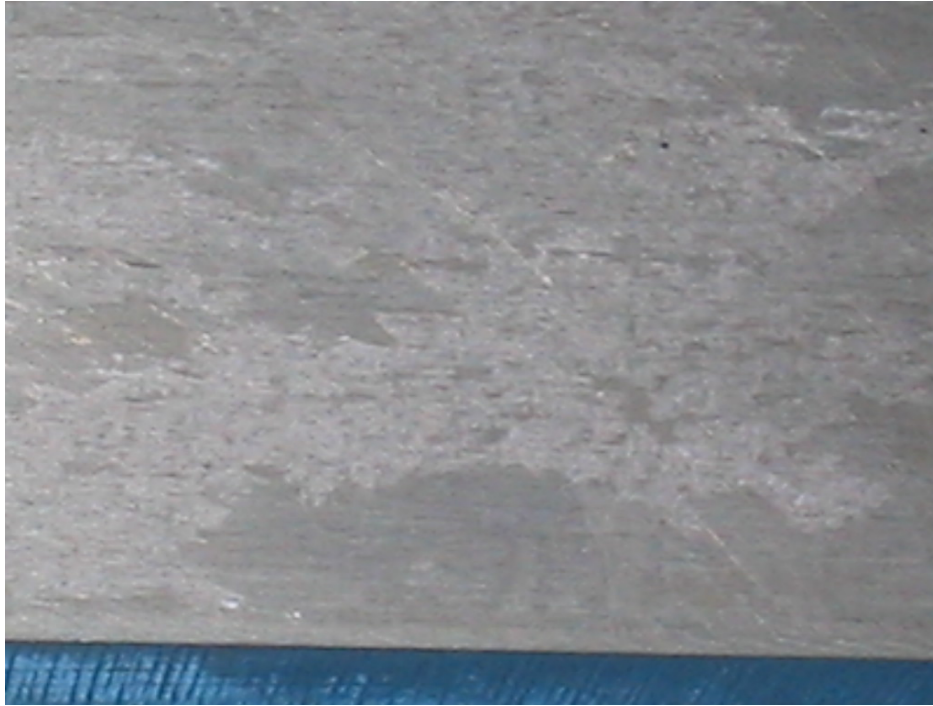
Figure 196. Close up of back of corroded and cleaned red notched beam
