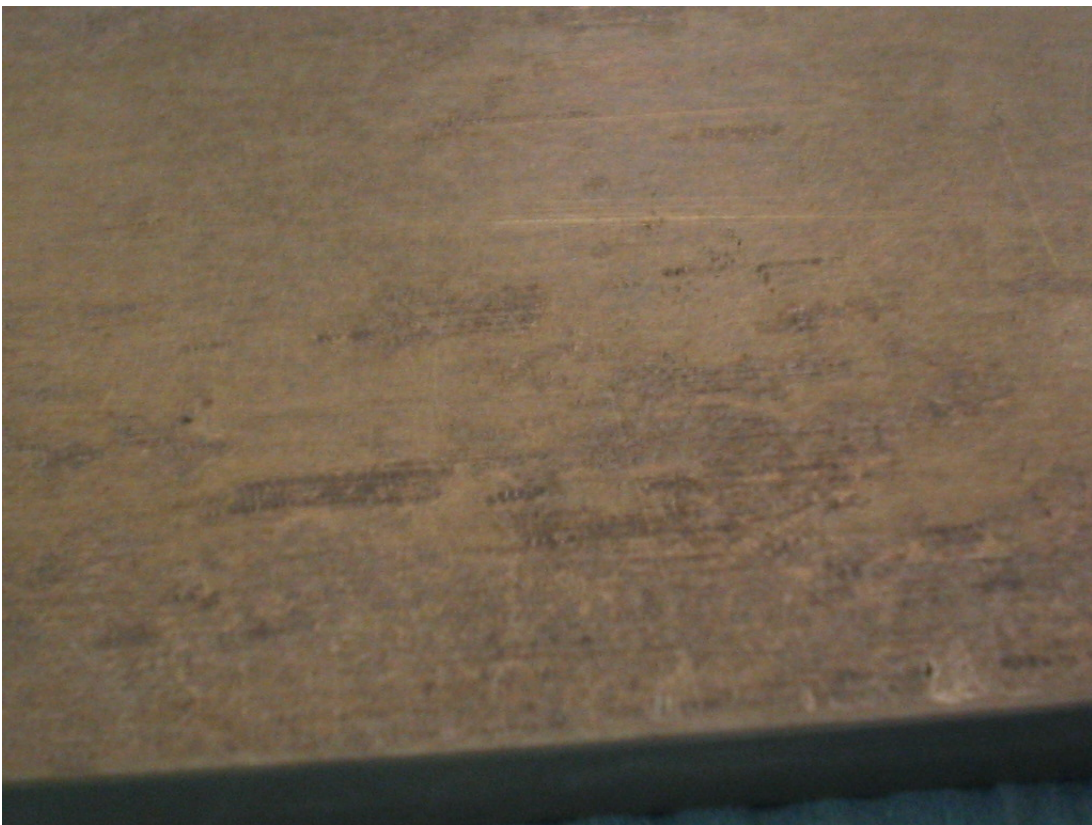
Figure 189. Zoom in on back of yellow cleaned beam. Overall corrosion and some apparent pitting despite the lack of salt deposits.
