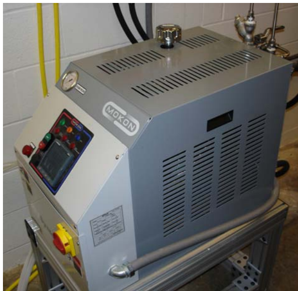
Figure 34: Mokon heater and pump unit for heat transfer oil used to cool emissions probe.
