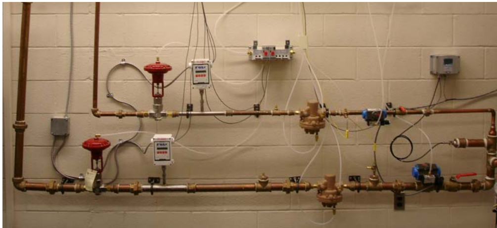
Figure 25: Rig airlines upstream of electric heaters.
