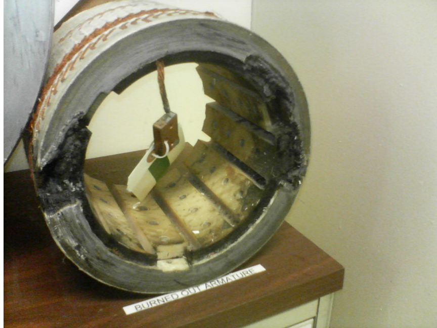
Figure 1. The armature from a liquid-hydrogen cooled generator. The rotors of the generator were high-purity aluminum which is a hyper-conductor. The windings of the armature are copper. Note the burned areas visible on the facing edge of the armature [7].
